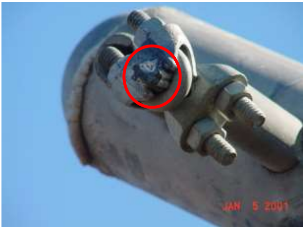
Figure 7.57. Evidence of arcing.
