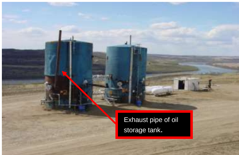
Figure 7.65. Oil storage tanks and exhaust pipe.
