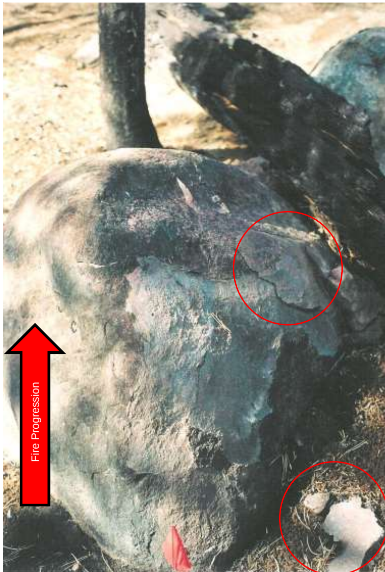
Figure 2.46. Example of spalling.
