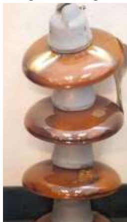
Figure 7.47. Evidence of arcing on a damaged insulator.
