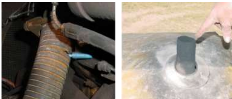
Figure 7.16. Damaged exhaust systems.
