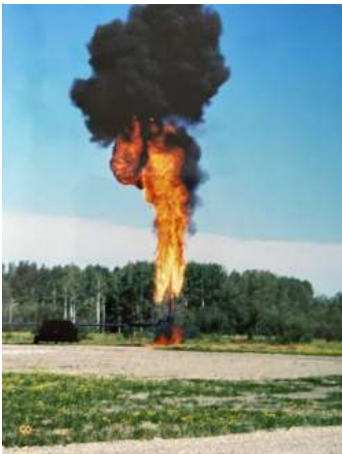
Figure 7.64. Malfunctioning flare stack.
