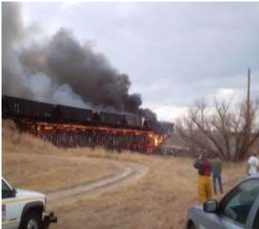
Figure 7.72. Railroad trestle fire.
