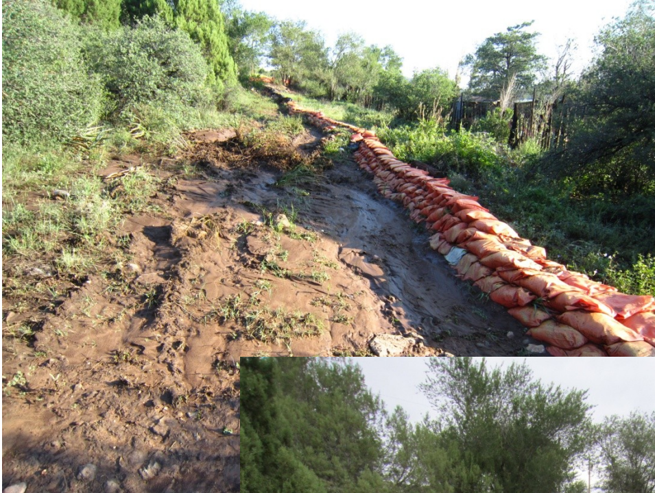
After first three storms too much sediment was building up behind sandbags.
