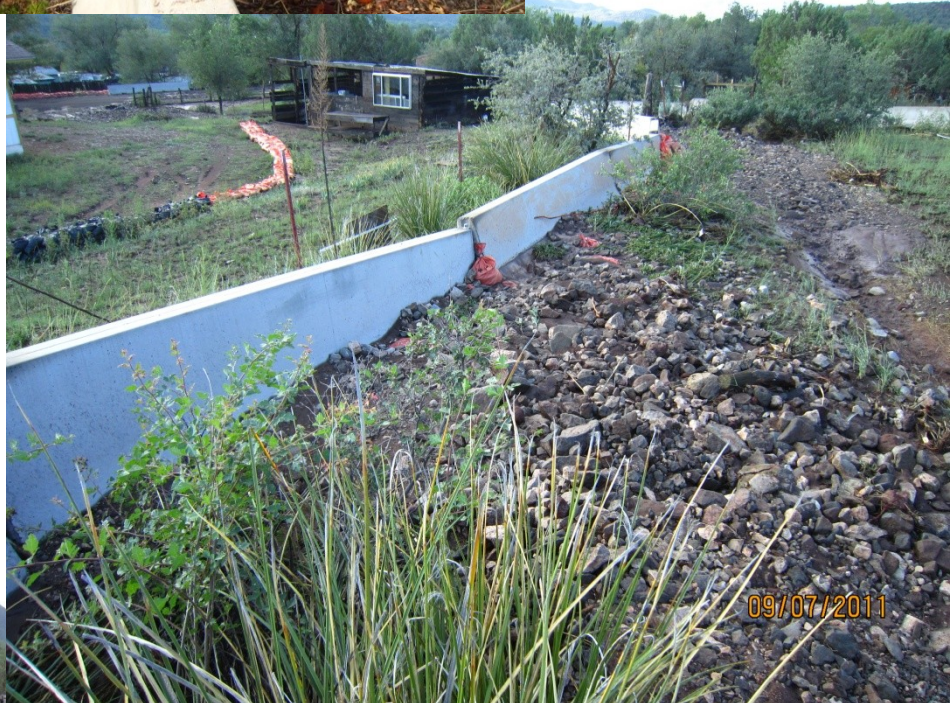
Behind k-rail after 9/6/2011 storm. Too much rock and sediment.
