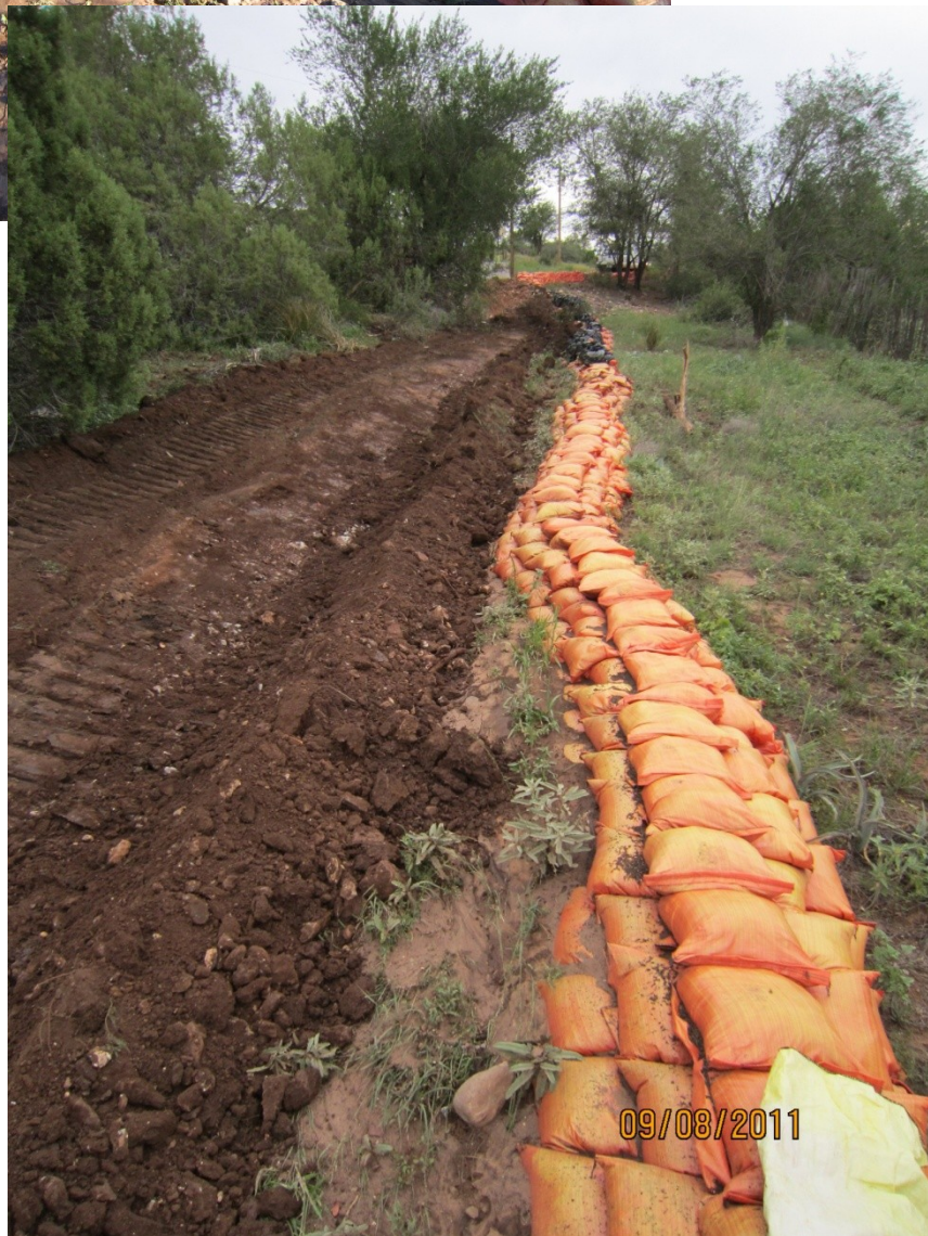
Solution after 9/6/2011 storm was to remove sediment and improve drainage before major flooding occurred.
