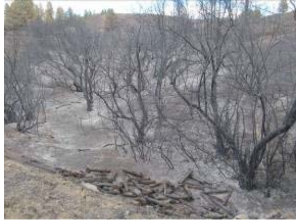
Burned pre-fire log jam above culvert along Elijah Road.
