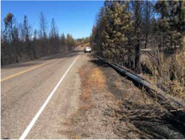
Damaged guard rail on Sherwood Mine road
