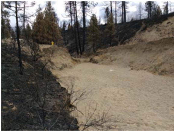
Bull Pasture road blow out from May 21, 2016 storm.
