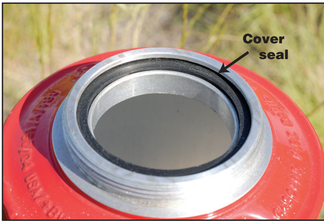
Figure 3-6—Inspect the tank cover seal for damage.
