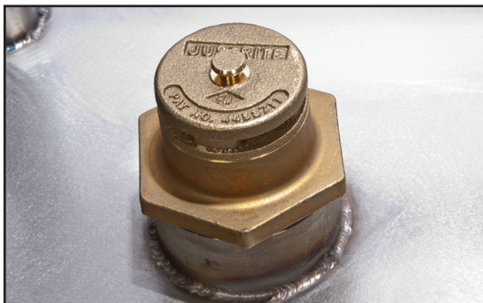
Figure 2-8 —This two-way tank vent prevents pressure or a vacuum from building up inside the tank. The vent has a flame arrester. Inspect the vent for external damage. Remove the vent to check for internal damage and clogging.
